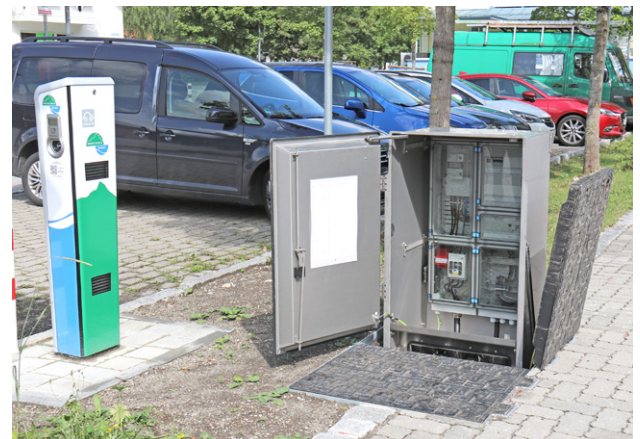
▲ EK880 charging infrastructure
