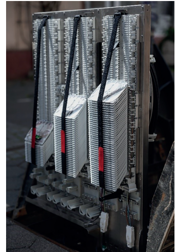
▲ Optical fibre underground distribution system with fibre management system folded open
