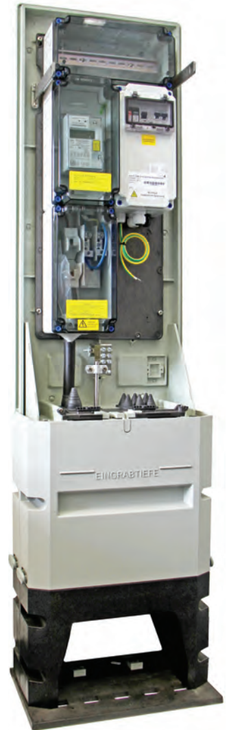
Example application: Power Supply Unit SVE 6 Z 129R installed in the energy terminal interface pillar EK 430
